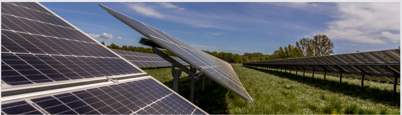
Photo by C4Energi
